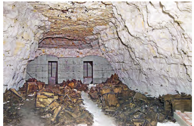
Main repository chamber with the remains of rotten tea chests used to store records in, and with the two vaulted secure stores at the rear
